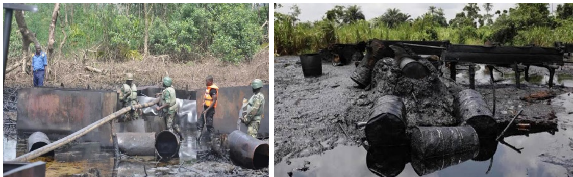
Figure 1. destruction of illegal refinery by security agencies.
